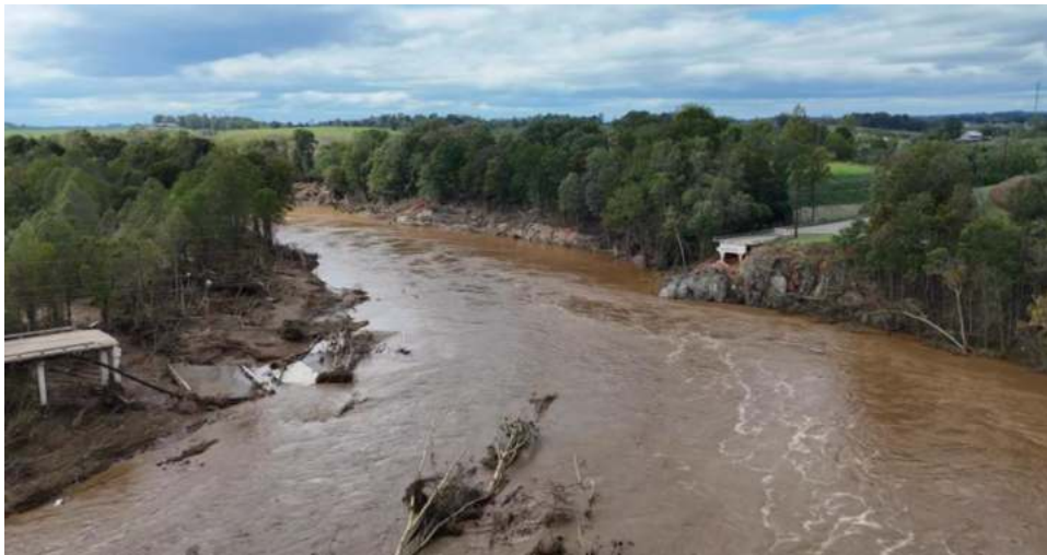
Remains of the Kinser Bridge on Hwy 107 over the Nolichucky River in Greene County. Source: Facebook
