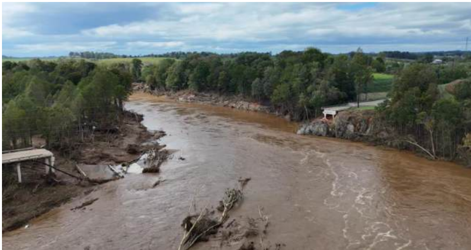
Remains of the Kinser Bridge on Hwy 107 over the Nolichucky River in Greene County. Source: Facebook
